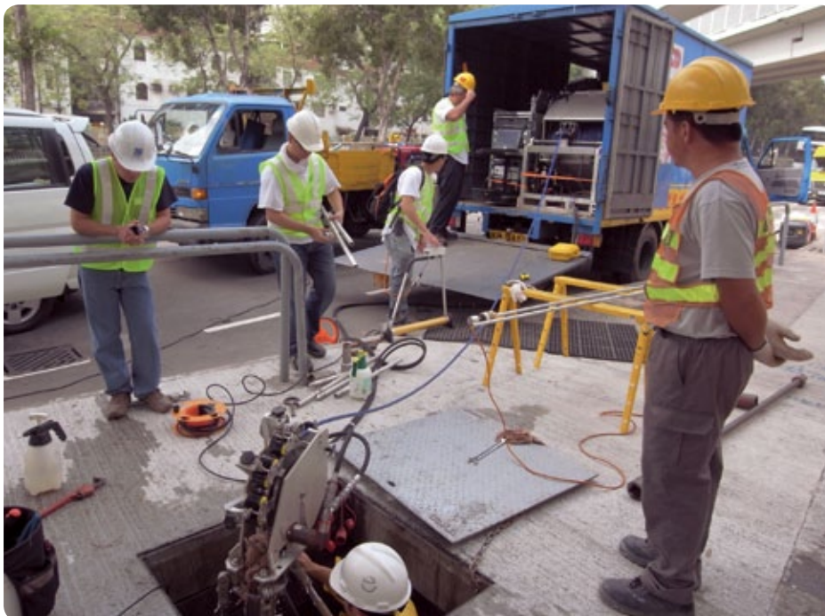
引入先進技術檢測運作中帶壓水管的滲漏情況。 A new technology is introduced to detect leakage in in-service pressurised water mains.
