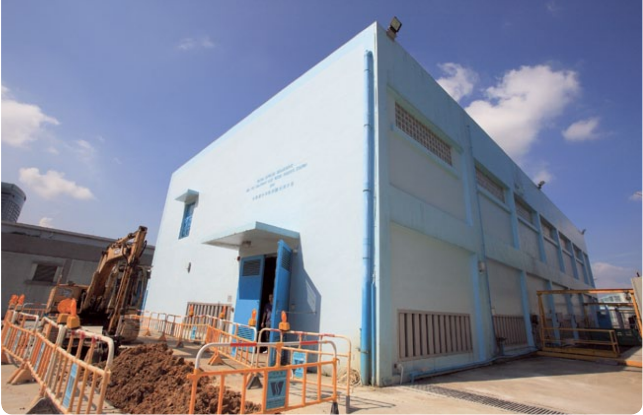
建造沙田海傍二號海水抽水站，提升沙田和馬鞍山地區的鹹水供應能力。 Construction of Sha Tin Seafront No.2 Salt Water Pumping Station will increase the capacity of salt water supply in the Sha Tin and Ma On Shan areas.
