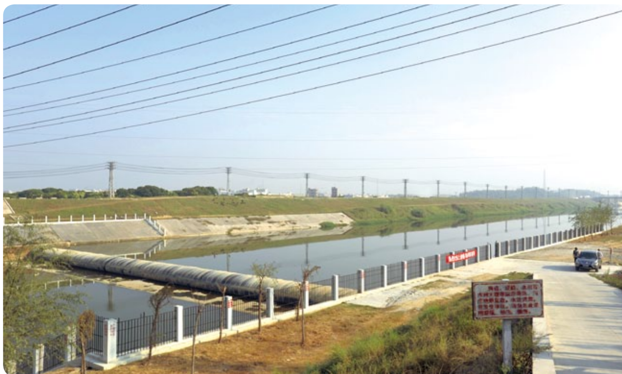
廣東省為石馬河進行調污工程。 Diversion of polluted water from the Shima River by Guangdong authorities.
