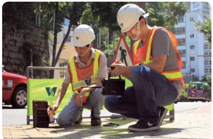
職員實地探測水管滲漏。 Our staff are detecting the leaks on site.
