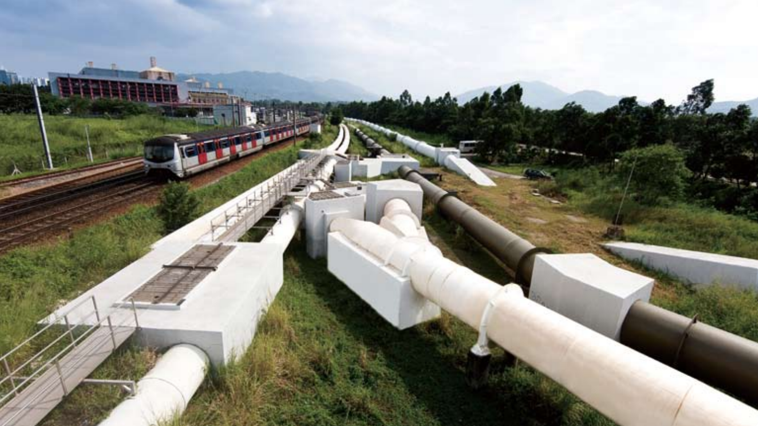
東江水為本港應付約七至八成的用水需求。圖示位於新界上水的東江水輸送管道。 Dongjiang satisfies about 70-80 per cent of our water needs. The photograph shows the water pipes for delivering Dongjiang water in Sheung Shui, New Territories.
