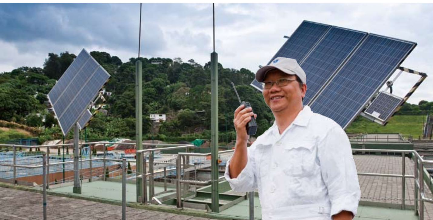
北港濾水廠率先試用太陽跟蹤光生電壓系統，效果理想。 A prototype sun-tracking photovoltaic system firstly used in Pak Kong Water Treatment Works has proved successful.
