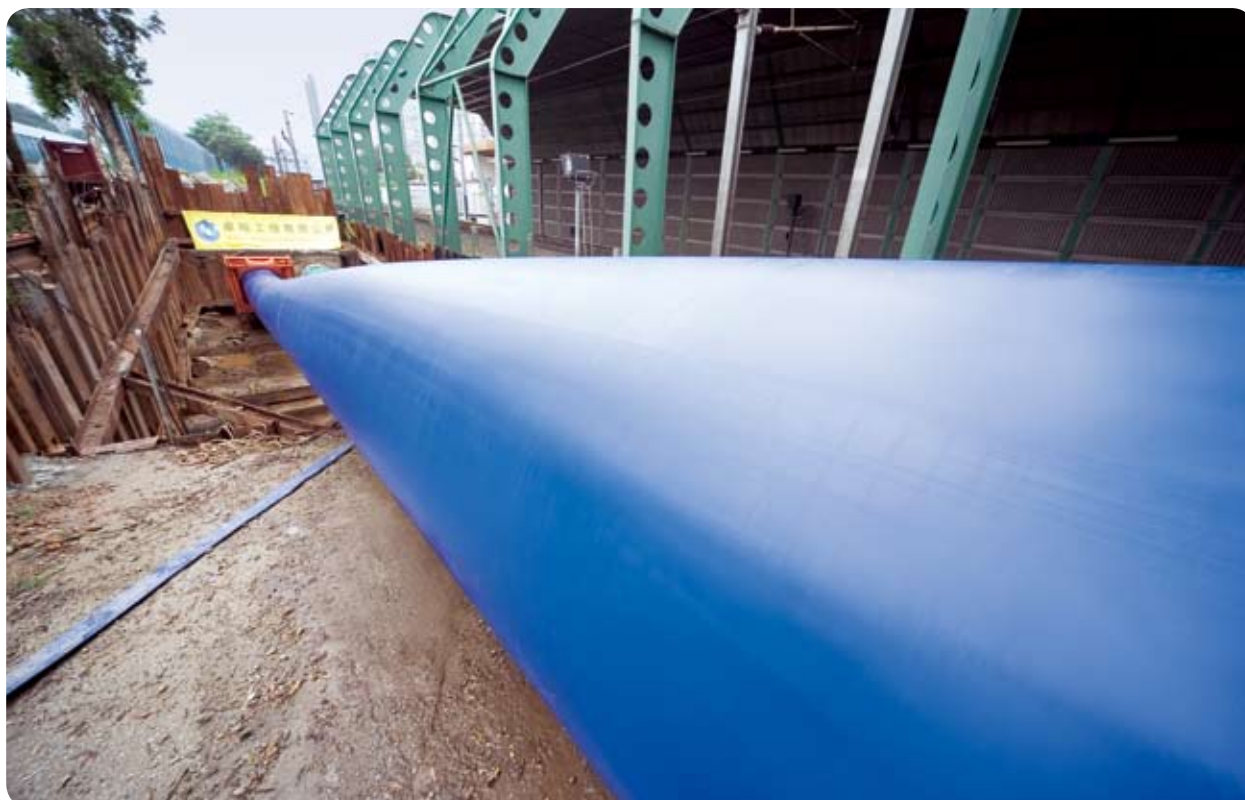
在粉嶺火車站附近，使用聚乙烯喉管進行大型水管的修復工程。 Rehabilitation of large water main with PE pipe near Fanling Railway Station.
