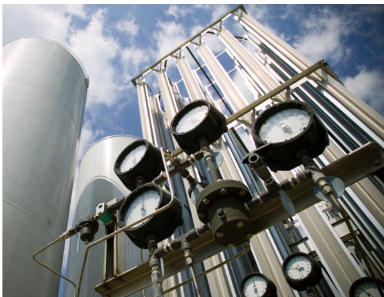
位於牛潭尾的氧氣儲存缸。 Oxygen storage tank at Ngau Tam Mei Water Treatment Works.
