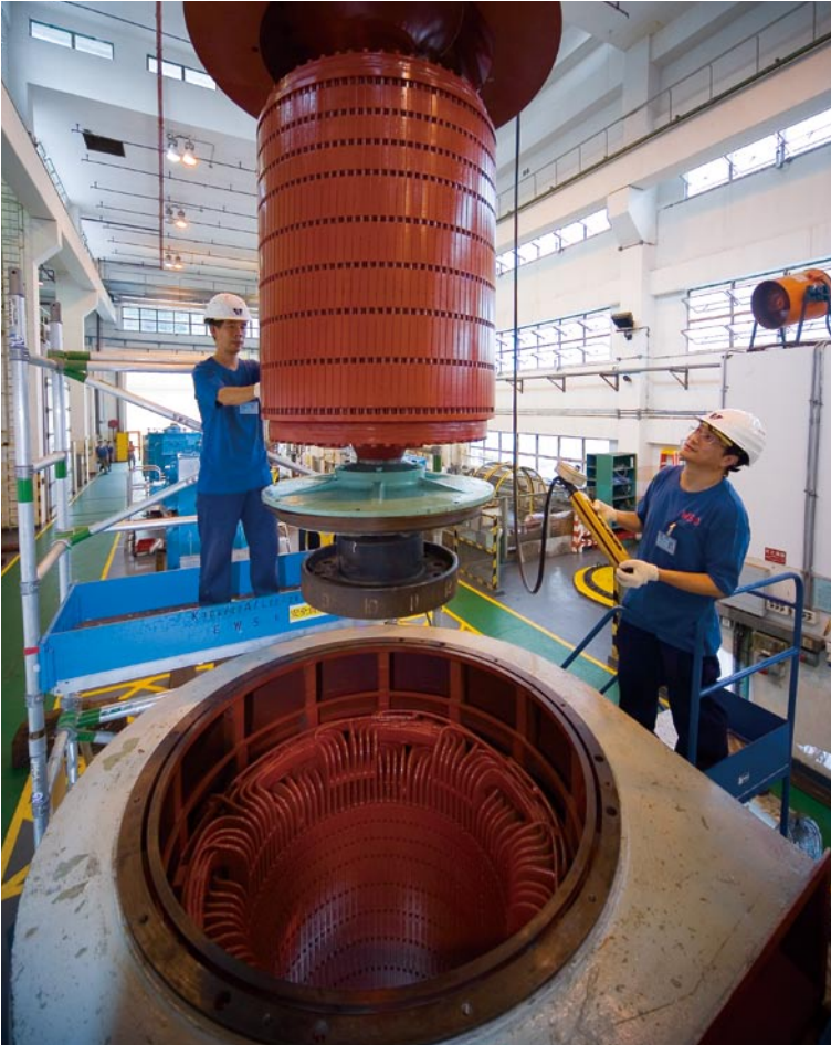
在龍翔道機電工場內為水泵的電動機進行維修。 Staff performing maintenance work on electric pump motor at Lung Cheung Road Mechanical and Electrical Workshop.
