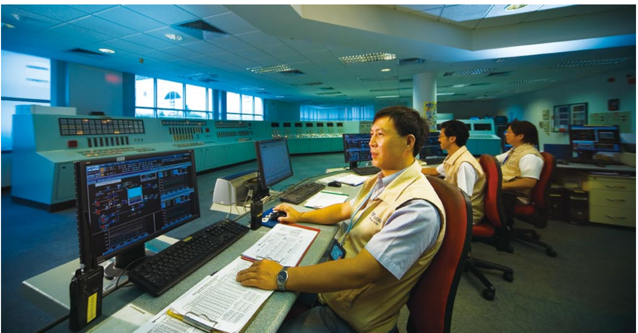
遙控濾水廠內設備的運作。 Performing remote plant operations at water treatment works.
