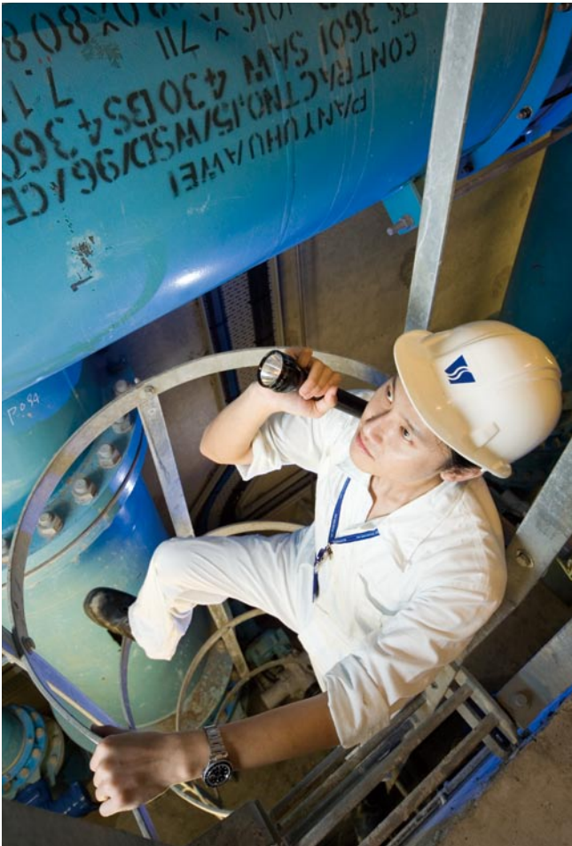
例行巡查對維持設備良好狀況是必要措施。 Routine inspection is necessary for maintaining the well being of plant.
