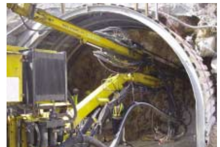
鑽石山二號食水配水庫的出水隧道正進行挖掘工程。 Excavation of outlet tunnel of Diamond Hill No.2 Fresh Water Service Reservoir.
