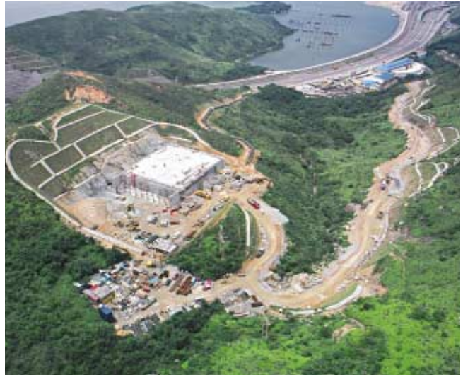
興建中的陰澳篤食水配水庫。 Yam O Tuk Fresh Water Service Reservoir under construction.
