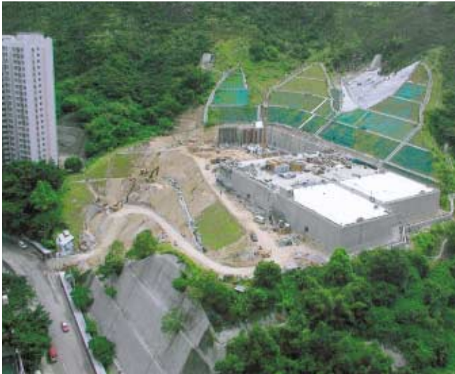
興建中的油塘二號食水配水庫。 Yau Tong No.2 Fresh Water Service Reservoir under construction.
