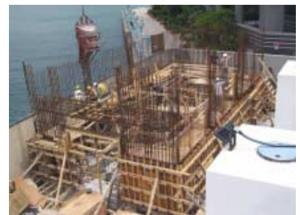
興建中的大環海水抽水站電解氯氣機房。 New Electrochlorination House of Tai Wan Salt Water Pumping Station under construction.
