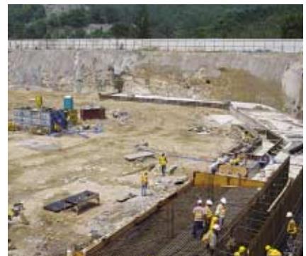
興建鑽石山二號食水配水庫的工地。 Construction site of Diamond Hill No.2 Fresh Water Service Reservoir.
