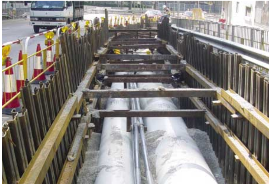
大型的地下食水和海水管道敷設工程。 Laying of large fresh water and salt water mains.
