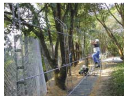
為水務設施安裝新保安圍網。 Erecting new security fencing for a waterworks installation.
