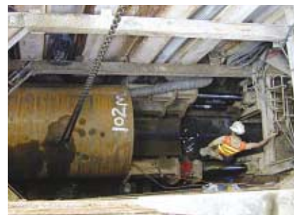
採用水管推頂方法於交通繁忙的道路敷設地下水管。 Using pipe jacking method to lay new water mains under busy road.
