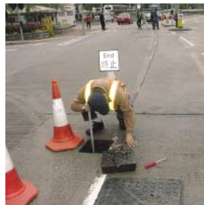
技術人員利用聽漏棍找出地下水管滲漏的位置。 Skilled staff using listening stick to detect leaks of underground water mains.
