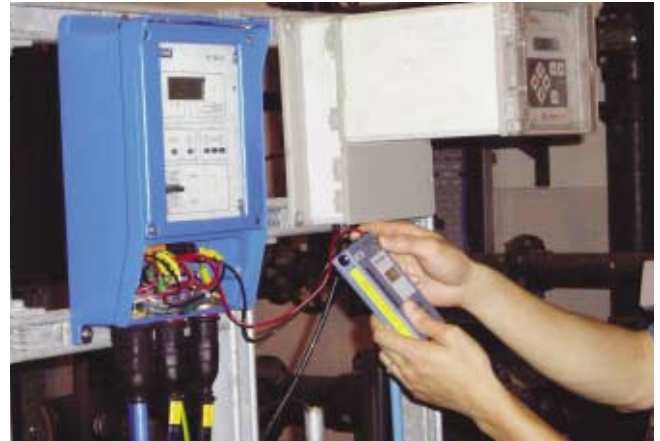
電磁流量計調校中。 An electromagnetic flowmeter being calibrated.
