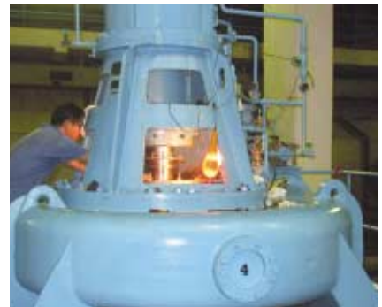
現場檢查和維修大型水泵。 A large water pump being inspected and repaired on site.
