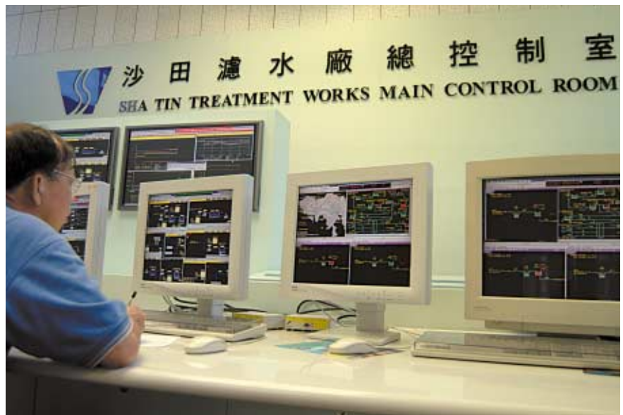
沙田濾水廠的「監控及資料收集系統」。 SCADA system at Sha Tin Water Treatment Works.
