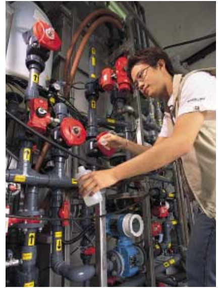
牛潭尾濾水廠內的超濾裝置。 Ultrafiltration pilot plant at Ngau Tam Mei Water Treatment Works.
