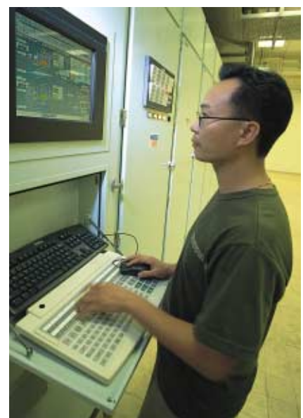
採用最先進的電腦科技控制濾水廠的運作。 Making use of latest computer technology for controlling operations of water treatment works.
