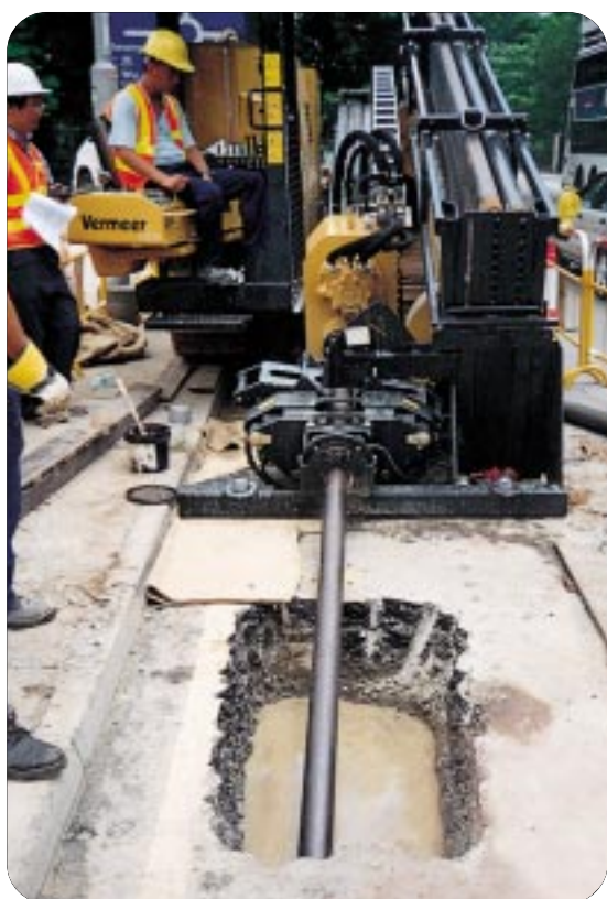
實地測試水平定向鑽控技術。 Trial test of horizontal directional drilling technique.
