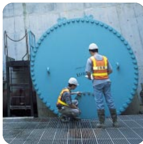
工作人員正檢查大埔濾水廠的水管。 Staff conducting inspection on pipework in Tai Po Water Treatment Works.
