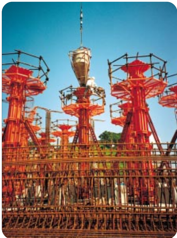
用以承托配水庫上蓋的支柱在建造中。 Columns for supporting the cover of service reservoir being constructed.
