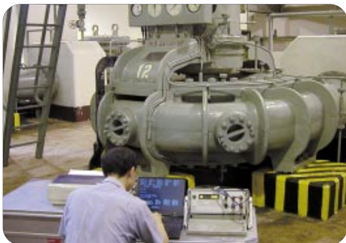
工作人員定期測試抽水機組的效率，藉以監察耗電量。 Staff conducting regular testing of pumpset efficiency to keep track of the energy consumption.
