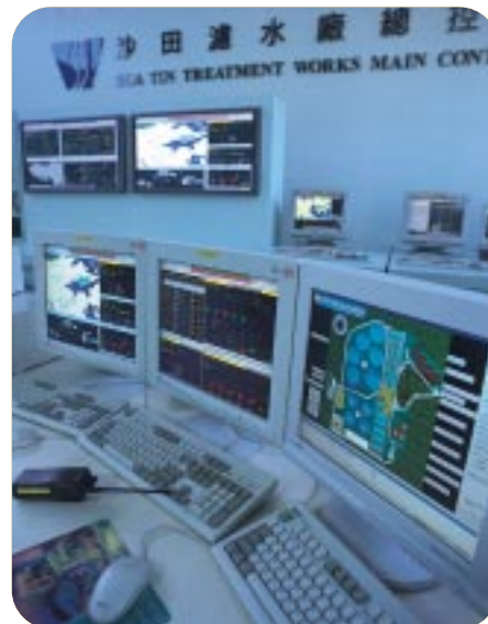
沙田濾水廠的監控及資料收集系統。 SCADA system at Sha Tin Water Treatment Works.
