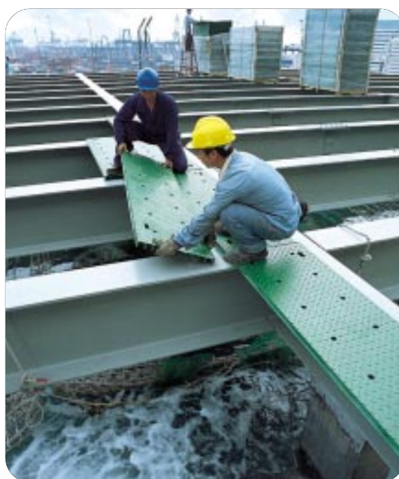
正進行海水配水庫的上蓋安裝工程。 Cover for a sea water service reservoir being installed.
