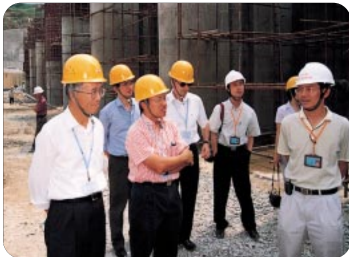
內地工作人員向水質事務諮詢委員會代表團簡介密封式輸水管道工程的進展。 Delegation of the Advisory Committee on the Quality of Water Supplies attending a site briefing of the progress of the closed aqueduct.
