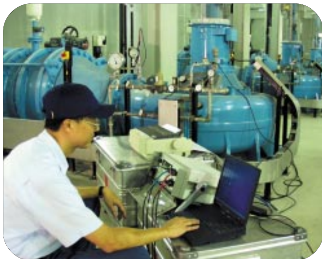
以最先進的儀器量度抽水機組的效率。 Using the advanced testing equipment for gauging the efficiency of pumpsets.
