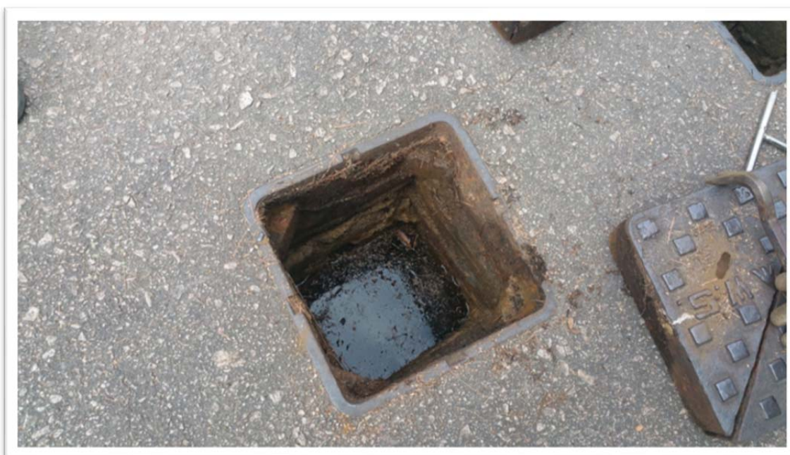
Photo 2 Valve pits flooded
