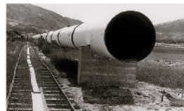
A large pipeline with a diameter of about 48 inches for the reception of water from the Shenzhen Reservoir.
