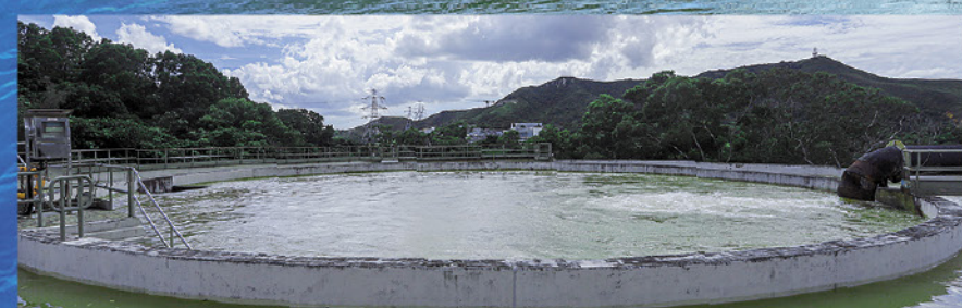
Sheung Shui Water Treatment Works Dongjiang raw water
