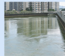
Dedicated Aqueduct - Jinhu Elevated Channel
