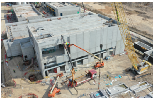
◆ 將混凝土外牆安裝至成品抽水站 Installation of external concrete wall panels onto the Product Water Pumping Station
