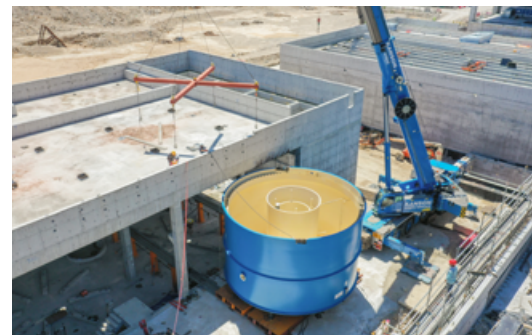
◆ 將熟石灰飽和器設置於後期處理大樓 Placing lime saturator in Post Treatment Building
