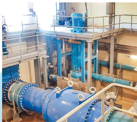
沙田濾水廠的水力發電站 Hydropower Plant at Sha Tin WTW
