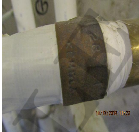
Photo 2. - Pipe Material / Copper / Kembla
