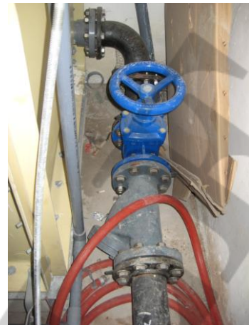
Photo 2. - DN80 outlet pipe
