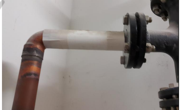
Photo 6 -67mm/ copper down pipe/Lawton
