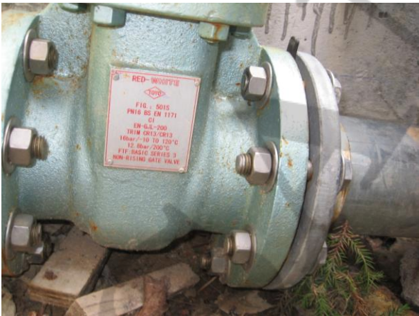
Photo 5 - Outlet gate valve / Toyo
