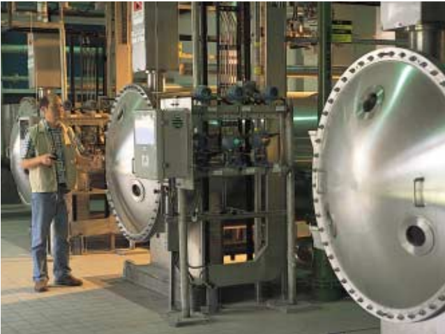
牛潭尾濾水廠內的臭氧生產器。 Ozone gas generators at Ngau Tam Mei Water Treatment Works.
