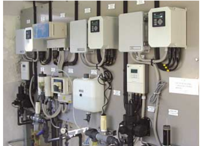
濾水廠內的聯機水質監察儀器。 On-line water quality monitoring equipment in a water treatment works.
