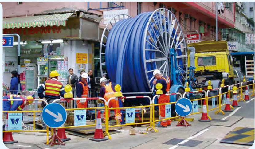
以「非開挖」方法修補水管。 To rehabilitate the pipeline by using trenchless method.
