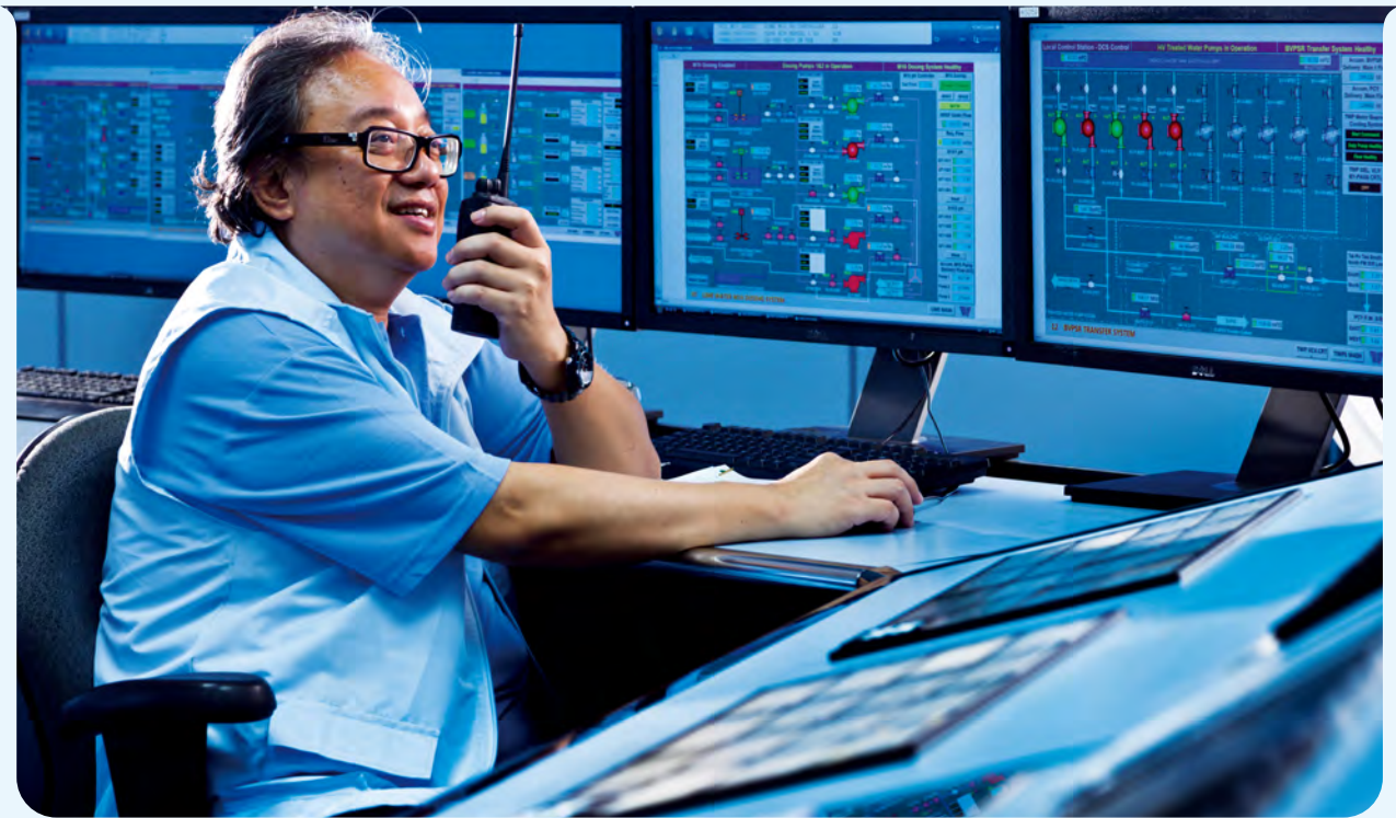
員工透過監控系統監察濾水廠運作。 Staff monitoring operations of water treatment works through the control systems.
