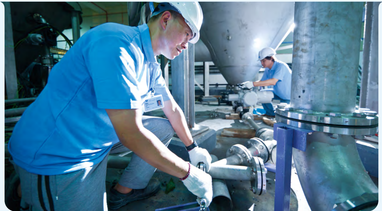
濾水廠內加建設施，提高生產力。 Additional facilities built in water treatment works to increase the capacity.
