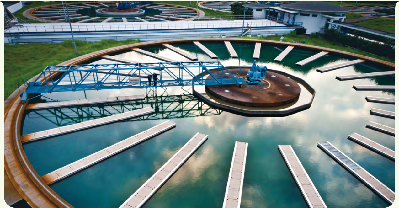
沙田濾水廠內的澄清池。 One of the accelerators in Sha Tin Water Treatment Works.
